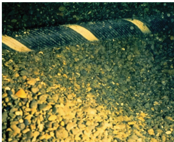
Figure 7.3 A power cable in the tide-swept Cook Strait, New Zealand, where currents move gravel (fragments >2 mm diameter) on a daily basis. Cables are protected by steel armoring with an outermost serving of polypropylene yarn, which is intact and retains its yellow-black markings after more than a decade of exposure to frequent sediment abrasion. (Photograph courtesy of Transpower New Zealand)
